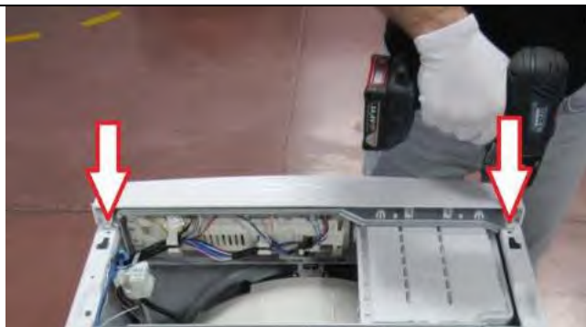
3.12 Tighten two screws fixing control panel.
