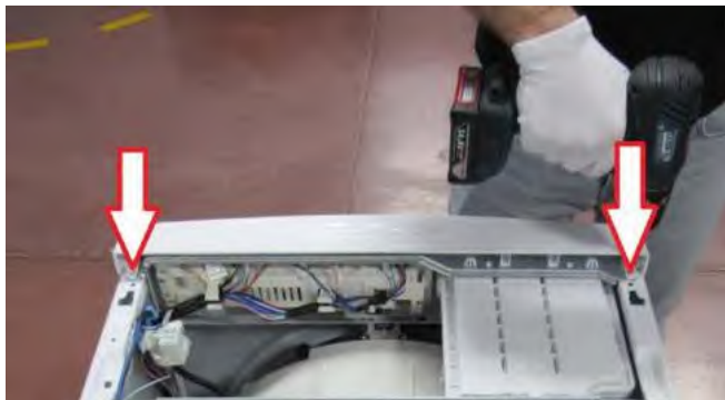
3.10. Tighten two screws fixing control panel.
